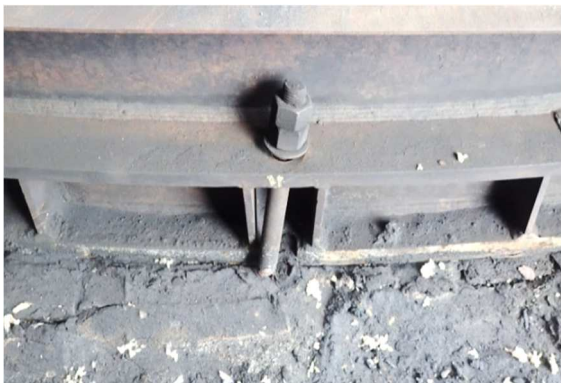
Figure 2 – Failure of Anchor Bolts
